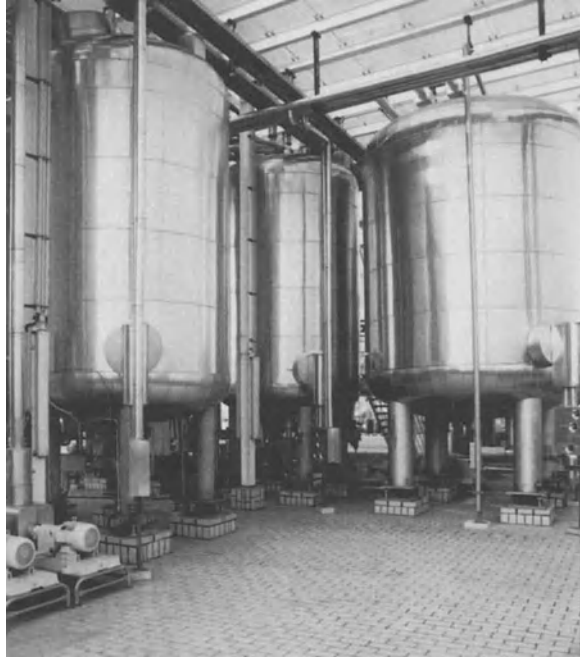
Fig. 6.91. Solvent tank farm with chemically resistant tile floor
