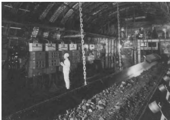
Fig. 6.189. Rubber conveyer belt in an underground mine
