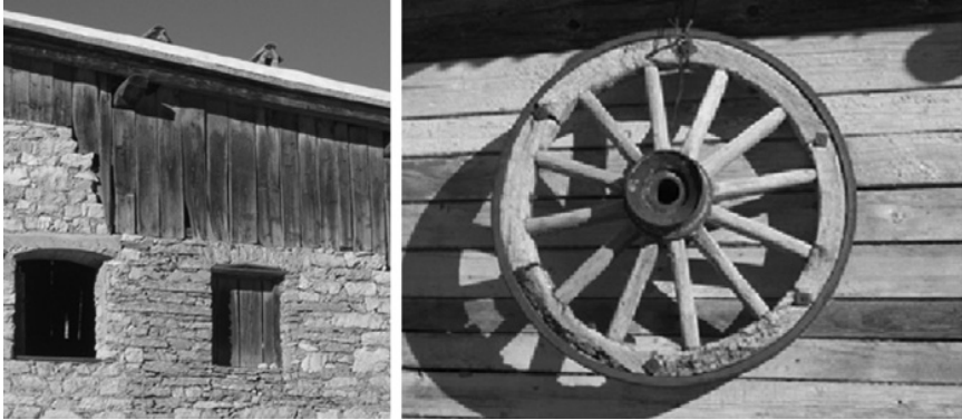
Figure 6 Examples of wood degradation.
