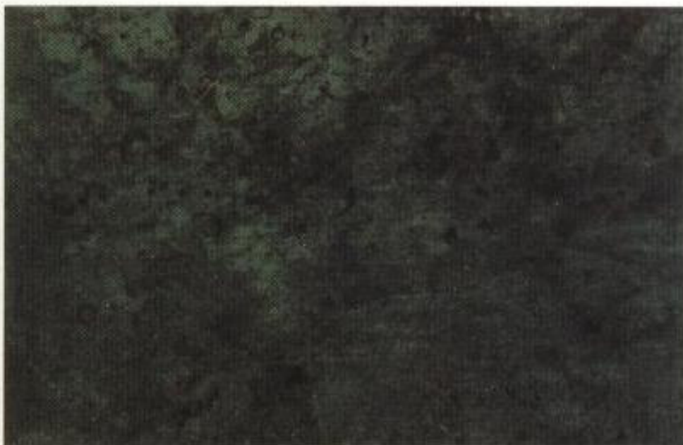
Steel surface largely covered with adhering mill scale but little, if any rust.
