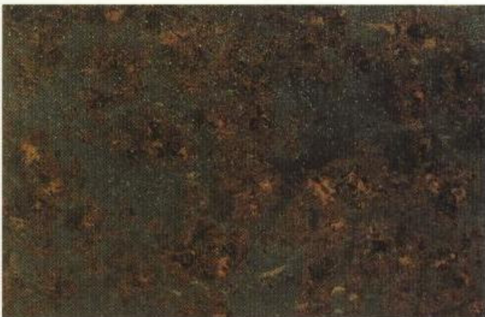
Steel surface which has begun to rust and from which the mill scale has begun to flake.
